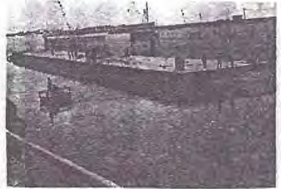
図 18 据付時水面に浮上したゲート(MSHI) Gate floating on water for installation (MSHI)
